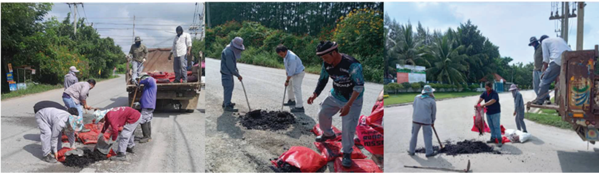
Participate in improving and repairing roads 3206(Wang Nam Chon) with Nong Makha Mong Subdistrict Administrative Organization.
